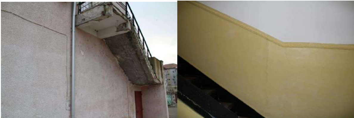
Fig.8 Some of the structural damages are visible
